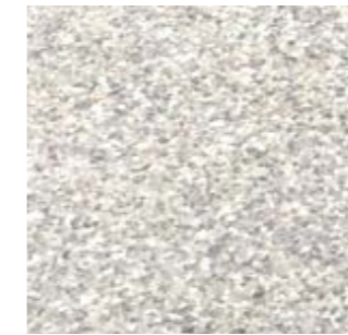
In-situ exposed aggregate concrete slabs To be used on or off-plot, and specifically on the dock edge. Vary movement joint grid dependent on location.
