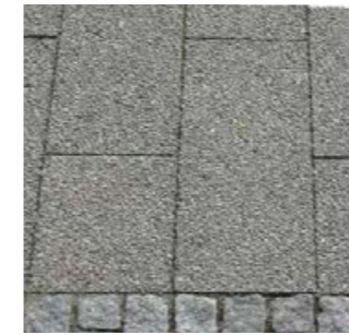
Exposed aggregate concrete slabs To replace existing only, where wholesale replacement of dock edge paving is not preferable.
